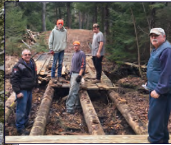
The Crankpullers' trail work crew preparing to re-deck a bridge with materials paid for by club members. Not all heroes wear capes: Dan, Dave, Sal, Bret and Cam at the Tucker Brook Bridge. Photo/Tom Johnson
