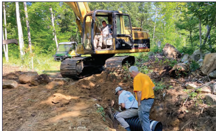
Don, Russ, Ryan and Steve install new culverts on the Homestead Trail on the Bridgewater Mountain system. Photo/Mike Phillips.
