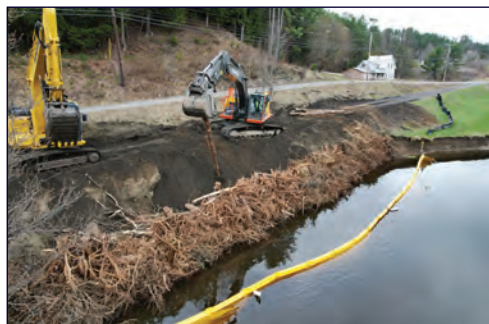
Root wads and logs are being installed into the bank to stabilize the trail.
